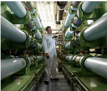
All Disney Cruise Line ships are equipped with Advanced Wastewater Purifications Systems.
